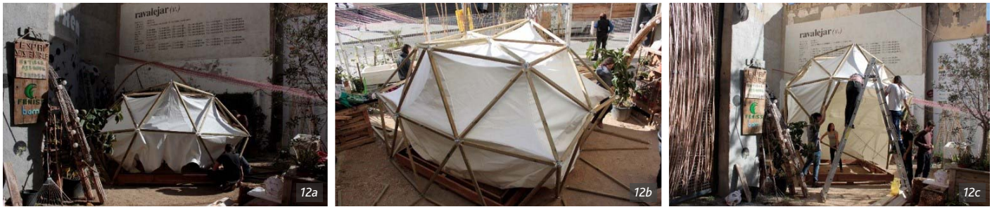
Figure 12a/b/c. Erection of the MH at the BAM BioBui(L)t -Espai Txema © Beatriz Arnaiz Barrio / LHRC Architecture Collective
