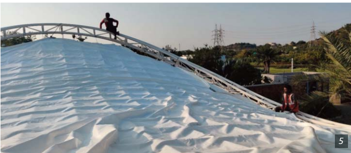
Figures 1-2. Front and side view of the entry canopy © SCHAFBOCK DESIGN WORKSHOP Figures 3-5. Erection process © SCHAFBOCK DESIGN WORKSHOP
